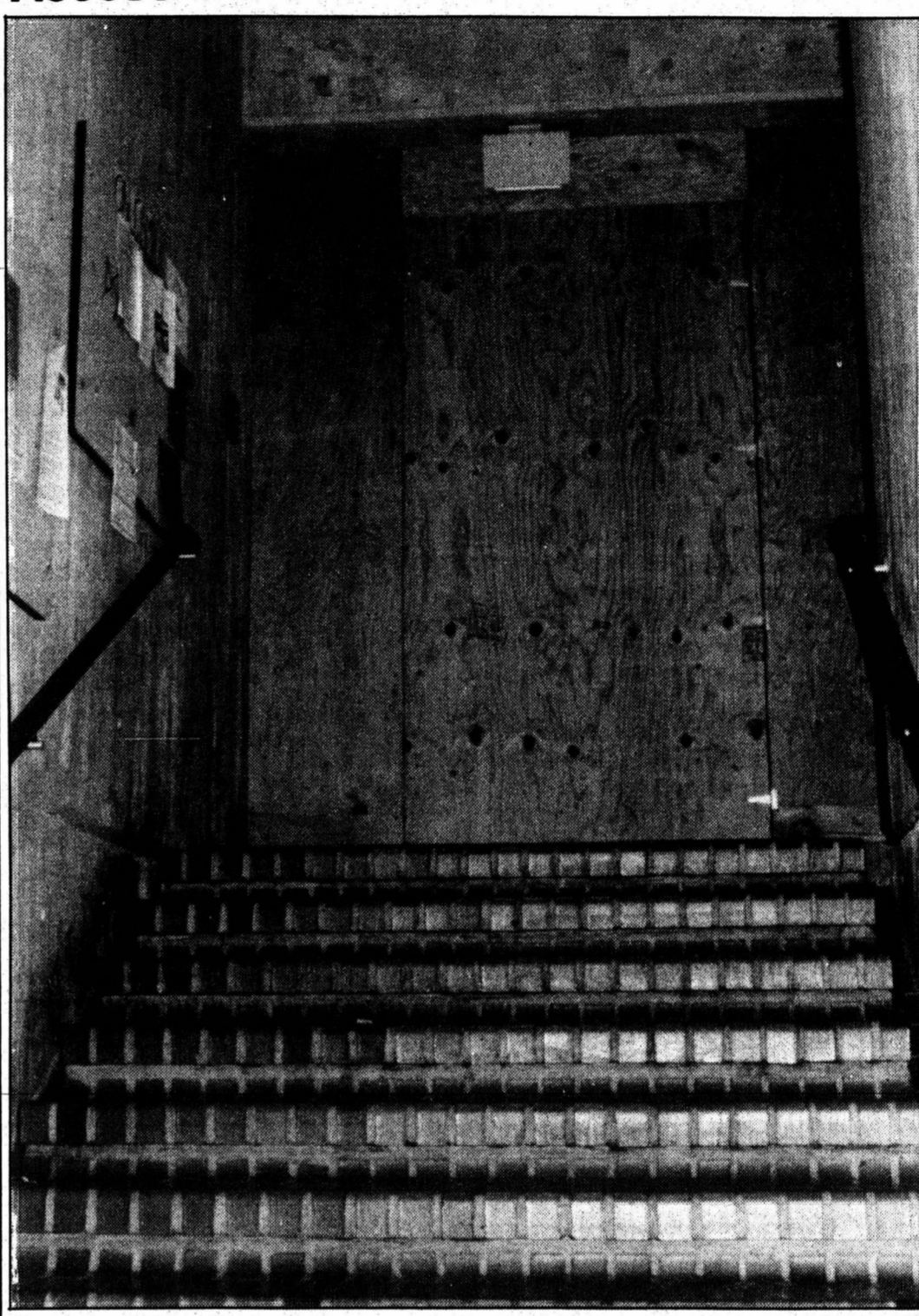
Students seeking an escape in the third floor of the Campus Activities Building have been greeted recently by barriers placed by construction workers. The Pit and other gathering places will be off limits until completion of the CAB expansion, scheduled for September. photo by Claire Littlewood
