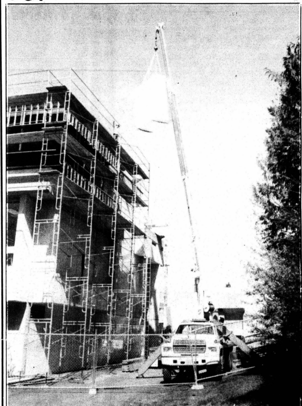
Although this looks like ozone-destroying polystyrene (aka styrofoam), it is actually CFC-free polystyrene for use as insulation in Phase II of the CAB. During the spring of 1989 a resolution was passed banning the use of CFCs and other ozone destroying materials at Evergreen whenever possible. photo by Tedd Kelleher
