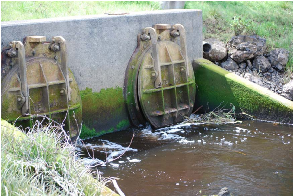
Figure 2.1: Tide Gate in Westport, Washington. Tide Gates Open and Close During Tidal Cycles Causing Intermittent Barriers to Stream Flow and Fish Passage.
