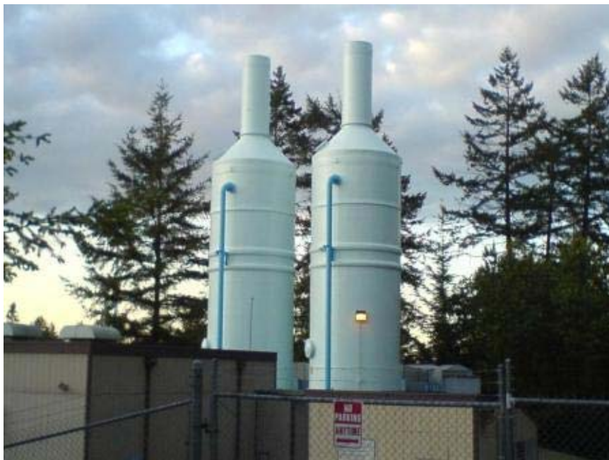
Figure 3-1 Air Stripping Towers. Photograph depicting two air stripping towers located in Tacoma, Washington. Source: Longley (2007)
