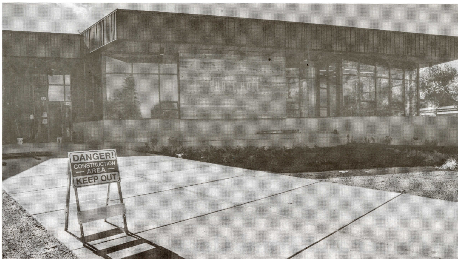
The new lecture hall remains under construction as school is about to begin. RICKY OSBORNE.
