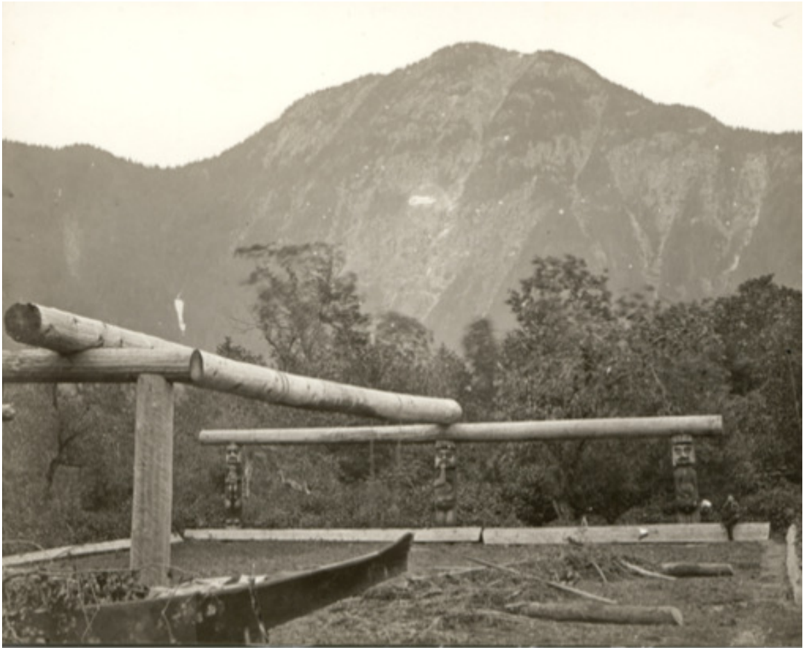
View of longhouse frame mid-construction. Kwakwaka'wakw (Kwakiutl) 1878, Vancouver, British Columbia, National Museum of the American Indian
