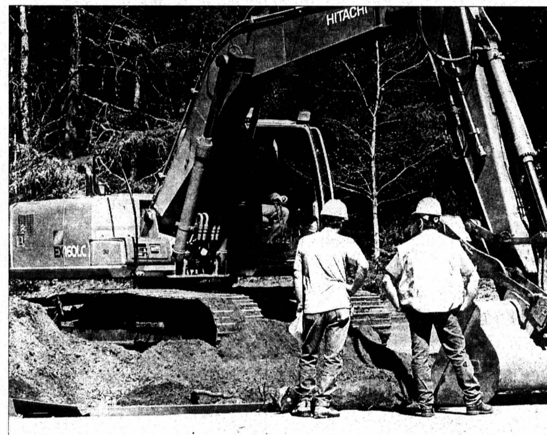
Construction for a one-lane roundabout begins on Evergreen Parkway. This project has faced opposition from some residents of Cooper Point Road, who have stated that "70 percent of the arterial use is through traffic," and the reduction down to one-lane is "unsafe and an ineffective use of funds." The Evergreen Board of Trustees approved this $1.5 million-dollar project in March.
