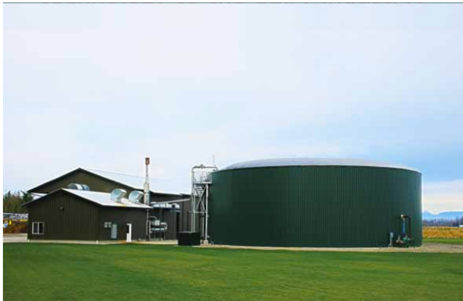
Figure 14. Van Dyk-S Holsteins Dairy digester facility, with generators in building on left; complete-mix digester with flexible cover for biogas collection on right (Daritech, 2011)
