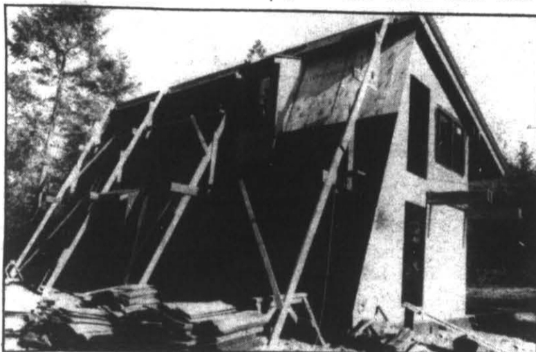
Construction of a local solar design house. Tours available over the weekend.
