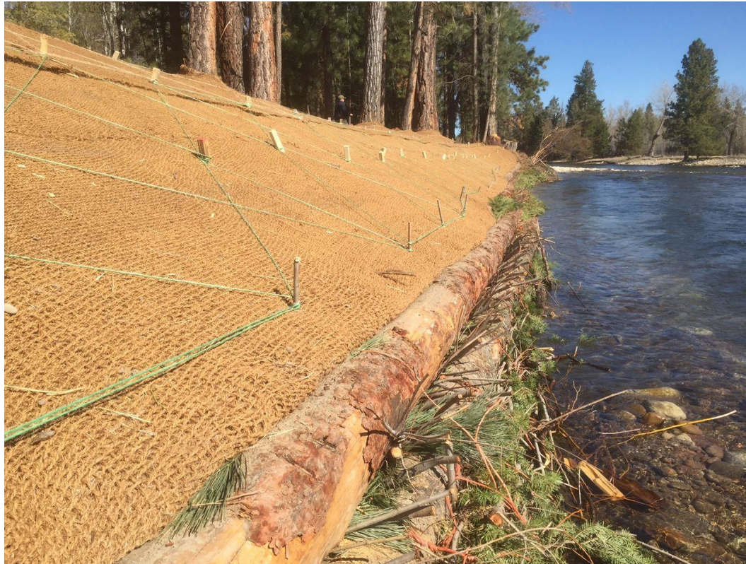
Figure 6.3 Matting can prevent erosion from occurring in projected locations predicted from the 2006 Hydrodynamic and Sedimentation Report, part of the 2009 Deschutes Estuary Feasibility Study. (Ridges of Restoration)
