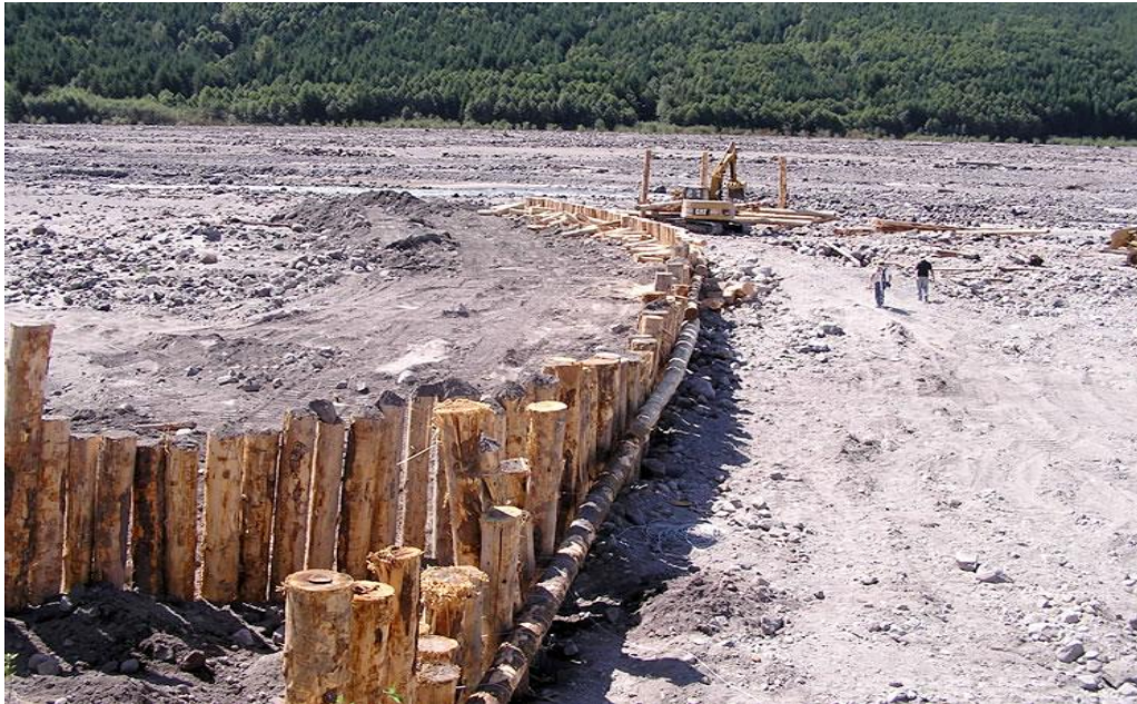
Figure 6.4 An example of a pile dike that can be placed throughout the Deschutes River to drop out sediment. (Mount St. Helens National Park)
