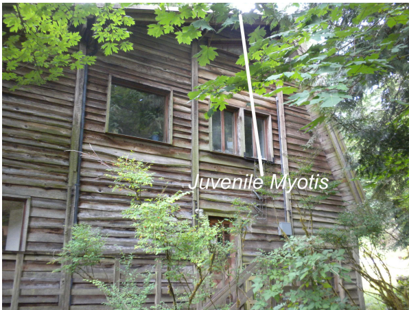
Figure 2. Juve. Myotis were observed roosting under metal roof flashing on the south side of the Farmhouse August 13.
