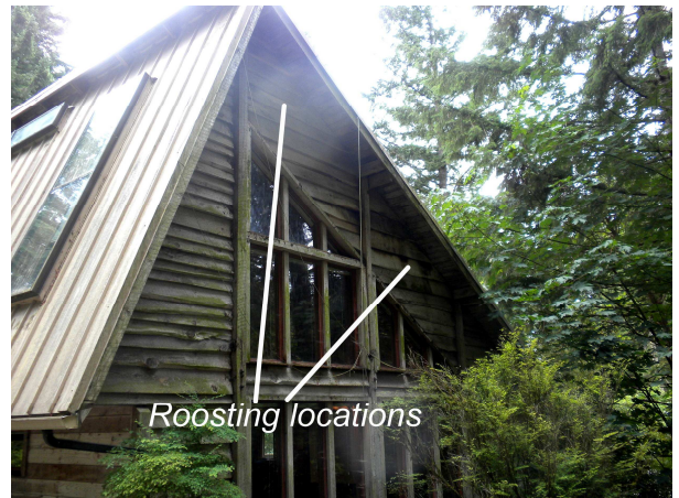
Figure 3. Two roosting locations were observed on the north wall of the Farmhouse. The area near the roof peak was used the most frequently.
