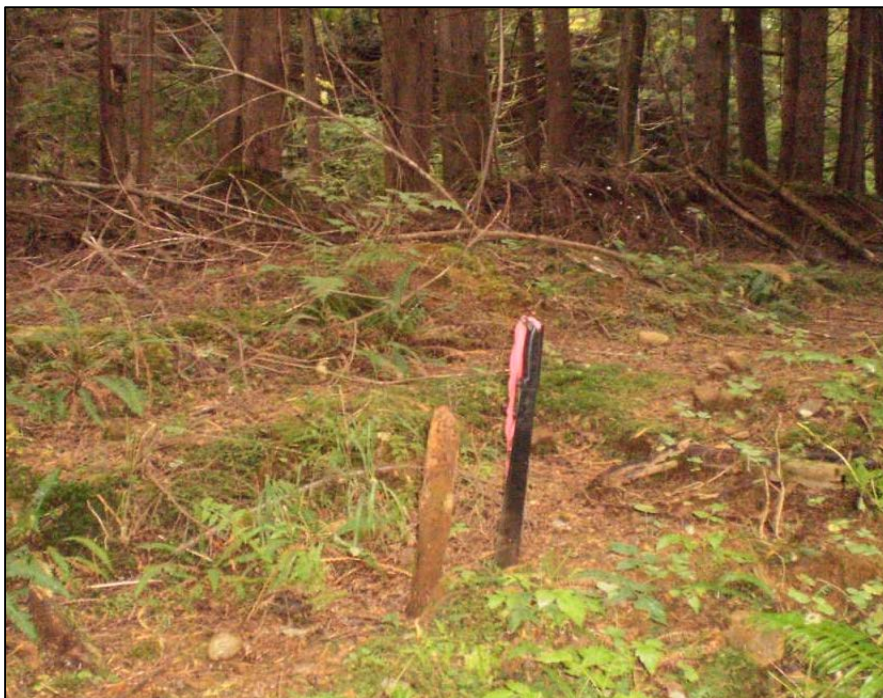
Figure 48. The 2-inch water pipe found in situ on a side grade above a deep through cut near segment J2. Photograph by author (Ferguson, 2012C).
