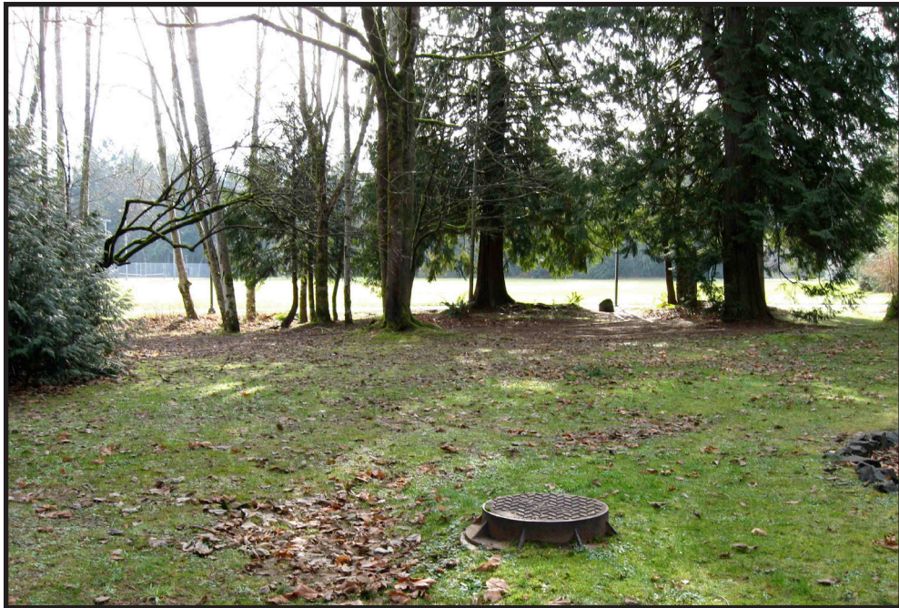
Photo 5.1 Before installation: looking southwest with athletic fields in the background. Photo credit: author.
