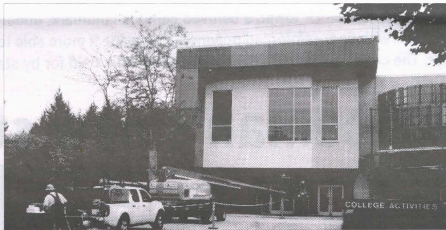
Construction was still under way into the start of the 2010-2011 school year. Archive photo
