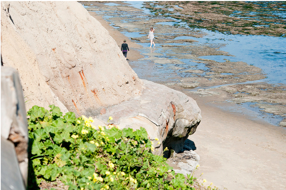
Figure 6. Pleasure Point Seawall Project corrosion structural failure.
