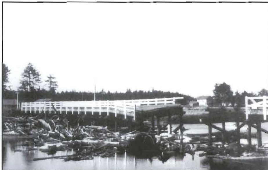
Figure 5: State Route (Highway) 109 @ Copalis River Bridge along the Washington coast showing massive damage from a tsunami event resulting from the 1964 Alaska Earthquake. Tsunami debris are lodged in and against the bridge footings from a 10-12 foot tsunami wave surge. (Tim Walsh, WA-DNR)
