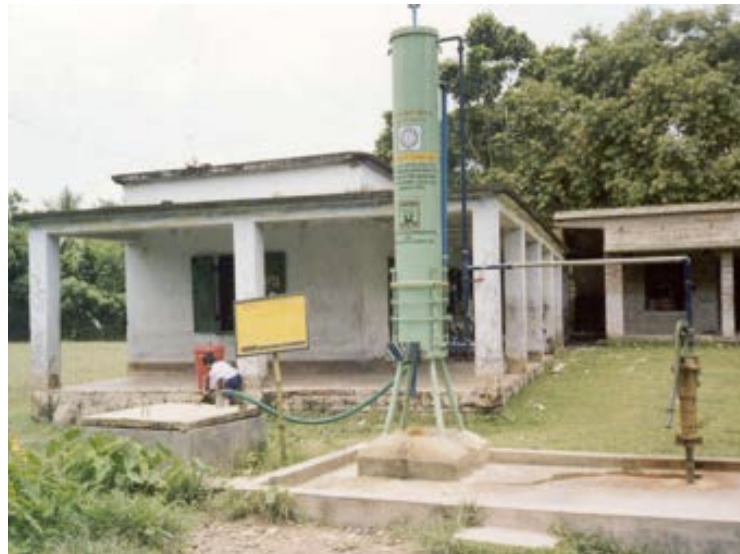
Figure 6 B: An Amal filter with the sludge pit to the left and the pump to the right (source: Bengal Engineering College)
