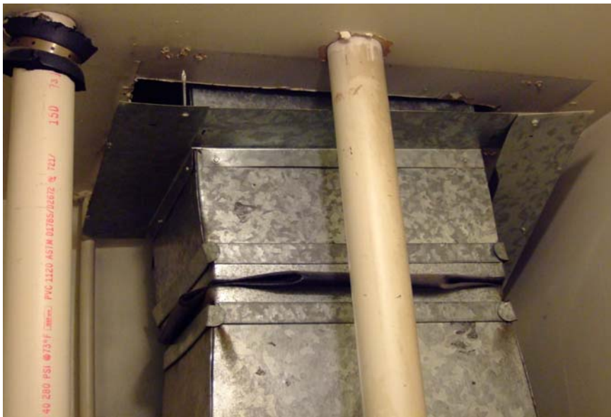
Figure 11. Furnace/utility room in unit Beachwood 8450
