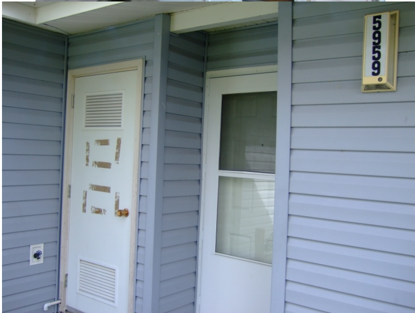
Figure 13. Utility Rooms: Louvre Door, units Davis Hill 5428 & 5959
