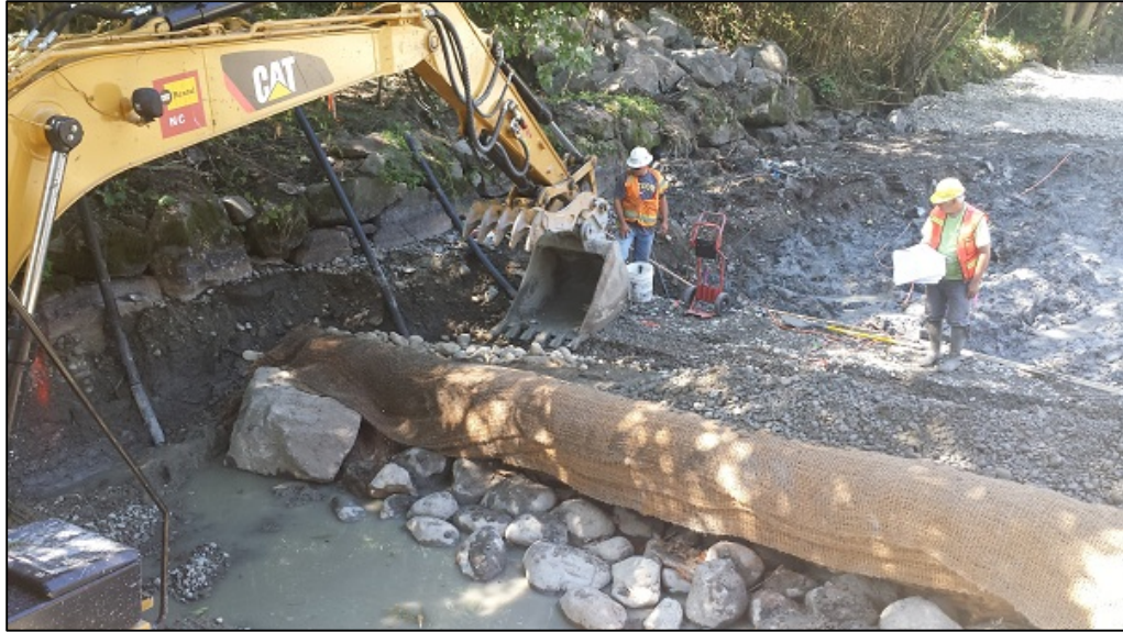
Figure 4: Photo shows the addition of a step-pool feature at the Knickerbocker treatment site. Also shows the constructed hyporheic substrate that consists of coarse sediment. Source: Seattle Public Utilities ( http://www.seattle.gov/util/EnvironmentConservation/Projects/KnickerbockerFloodPlain/index.htm )
