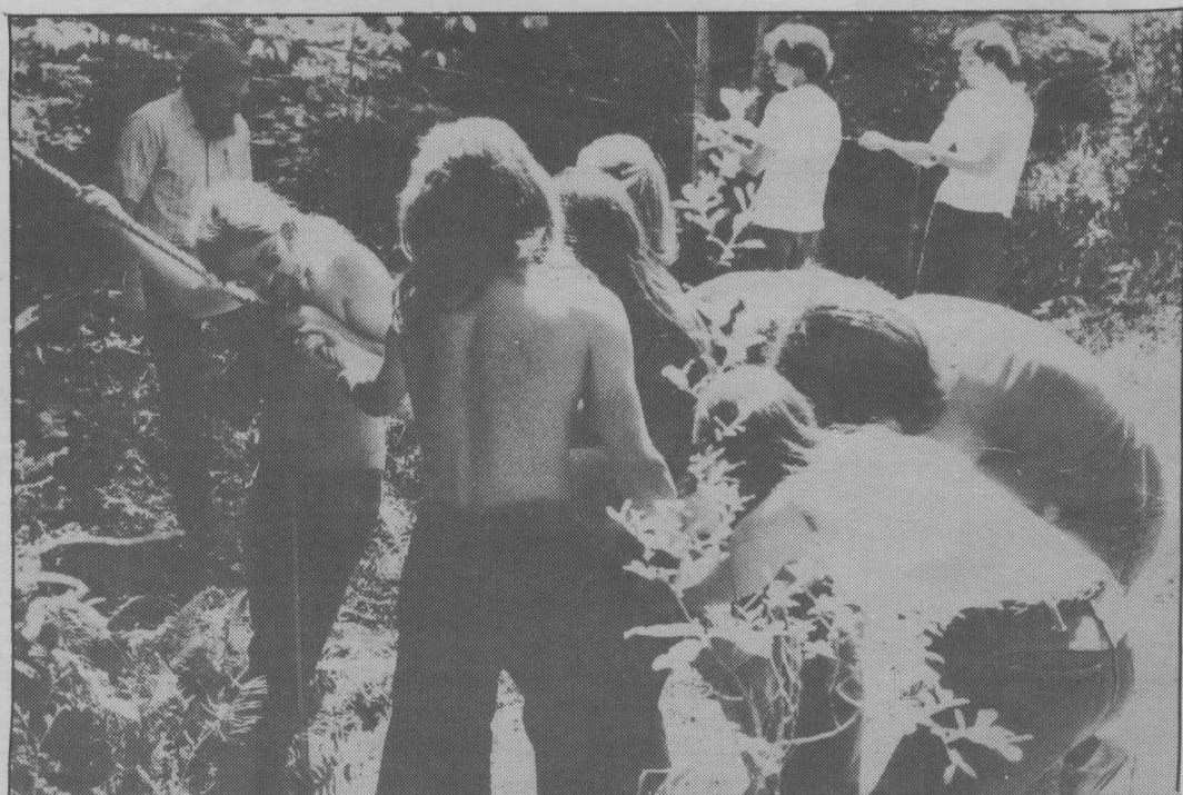
TOTE THAT LINE—Members of the Experimental Structure program erect Ichabod's pole. The first step in construction. (Photo by Gary Norton).
