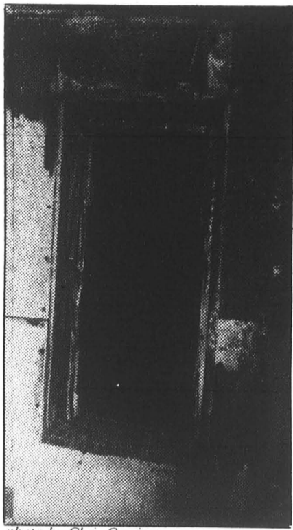
The metal frame of this window in C 314 was melted in last week's fire.
