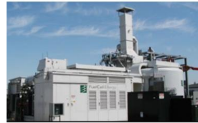
Figure 16: One-MW generator at King County South Treatment Plant (Source: King County Dept. of Water)
