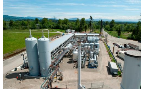
Figure 12: Cedar Hills Gas Processing Center (Source: Ingenco)
