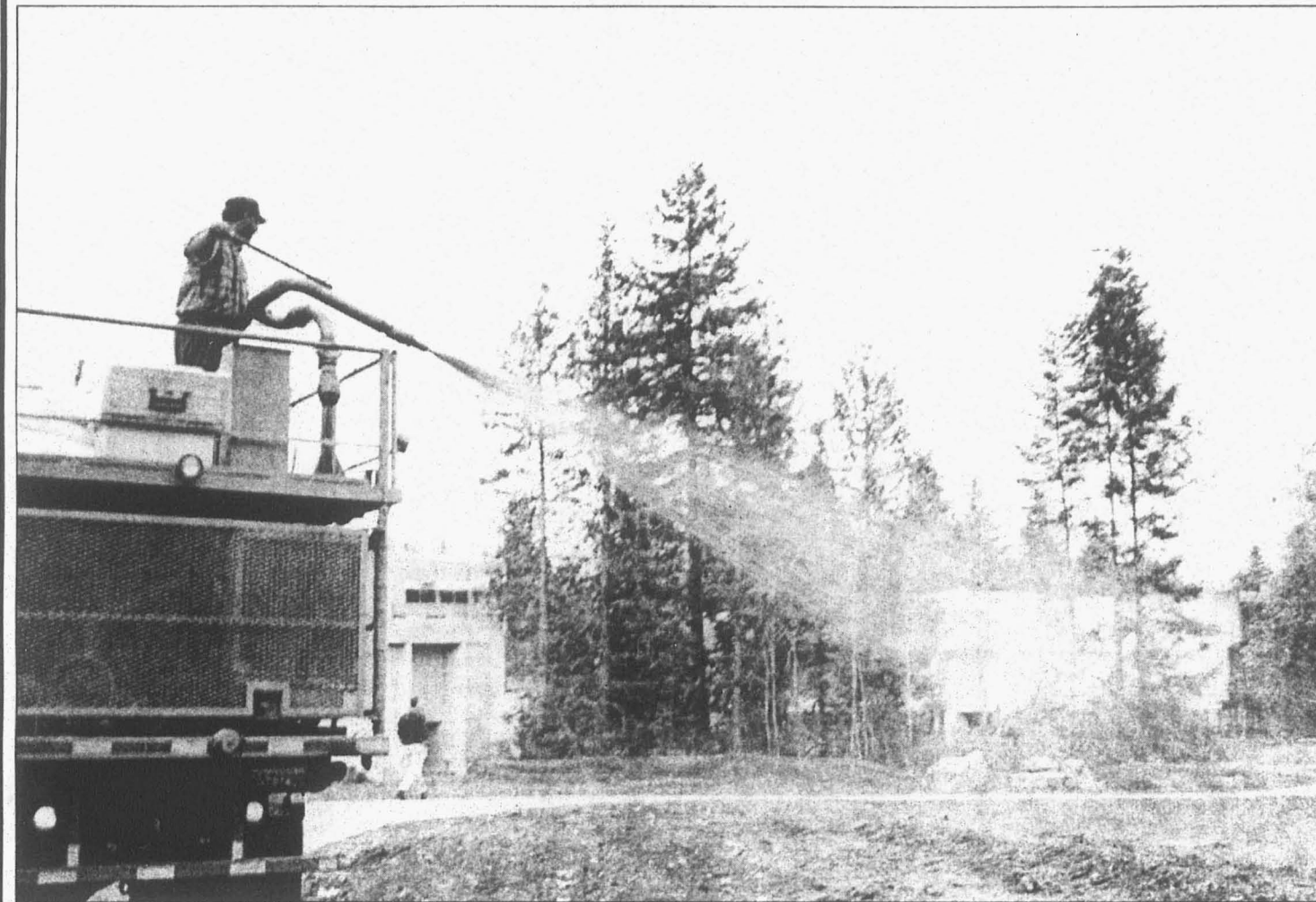
A worker with the Columbia Hydrosceding company, Wes Bodenhamer, sprays a mixture of grass seed, mulch, and fertilizer on the Seminar II site. Mark Kormondy, grounds supervisor with Evergreen facilities, says the "hydroseed" is intended prevent erosion. The hydroseed's bright green color comes from a dye. "Aesthetics isn't the issue," Kormondy said. The runoff from Seminar II flows into a local creek, and then to the bay. The future of the planned Seminar II building is still uncertain, as Evergreen waits for the Washington State budget office to release $41 million for the construction.
