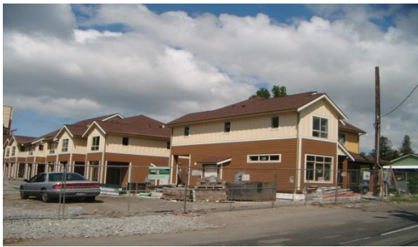
Figure 8: Photo of townhomes under construction at the Community Gardens at Rainier Court, Phase Three. Photo shows current conditions at time of research. 05/11/14.
